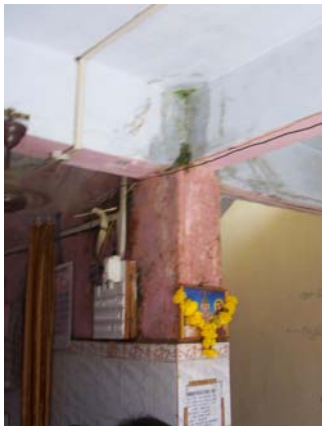
Figure 2 and 3: Anna Nagar SSP block showing critical water leakage in proximity to electrical installations but clean and well maintained toilets
